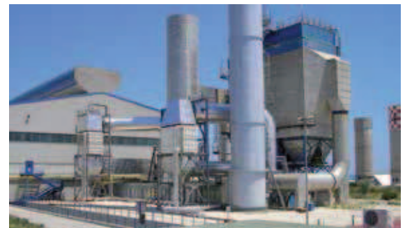
Figure 3: Flue gas treatment and heat exchangers at the Sangalli Manfredonia plant.
