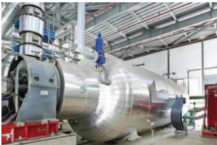
Figure 2: Organic Rankine cycle turbogenerator of the AGC Cuneo plant.
